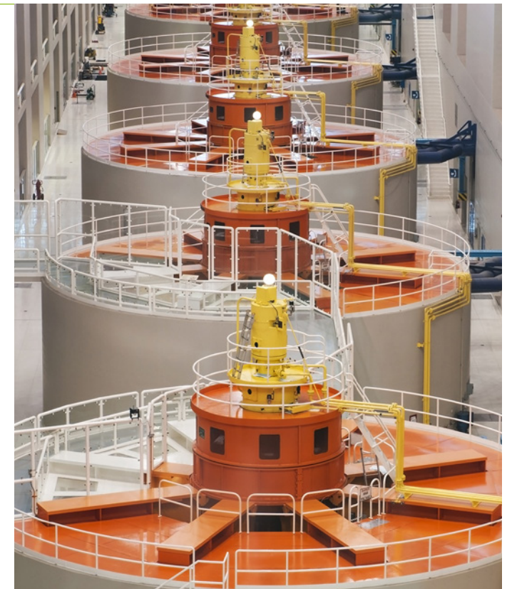
An example of a hydro power house, the Bonneville Dam on Columbia River, USA
